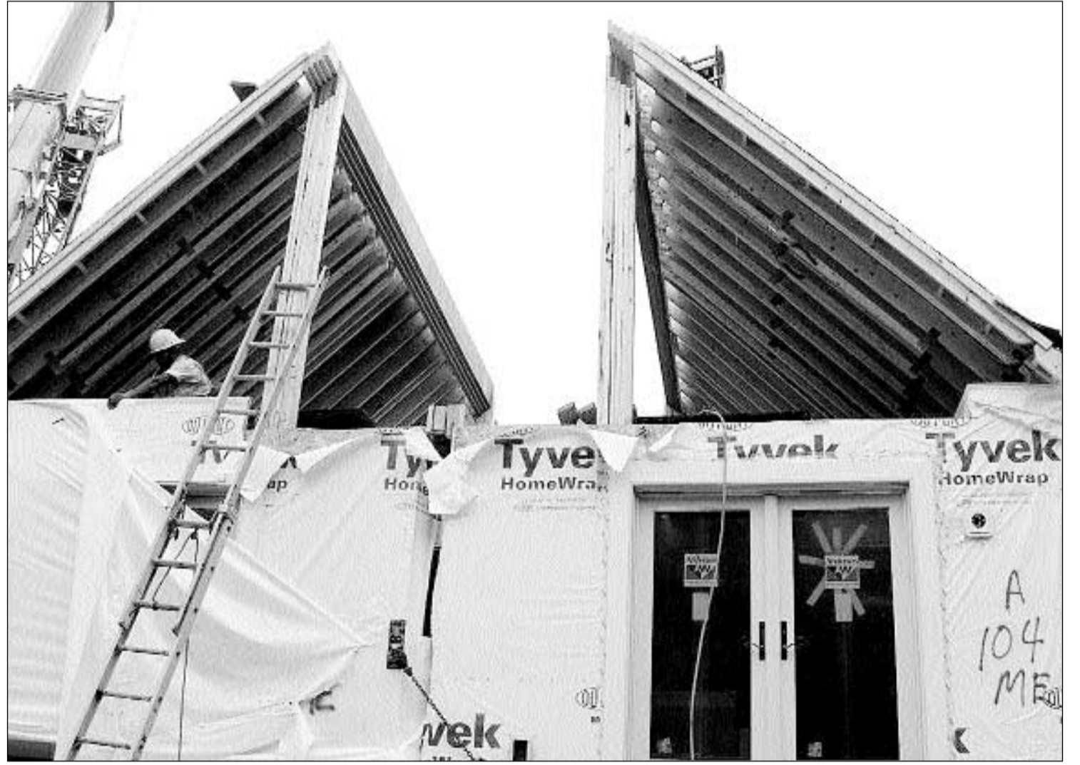
Builders leave room for a gable to be installed in the upstairs of the modular home being assembled in Owls Head by Bay Point Homes LLC of Rockland.
